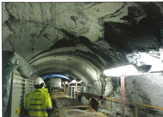
(c) New parallel TBM tunnel at the Lower Røssåga powerplant. Photo: Leif Lia.
